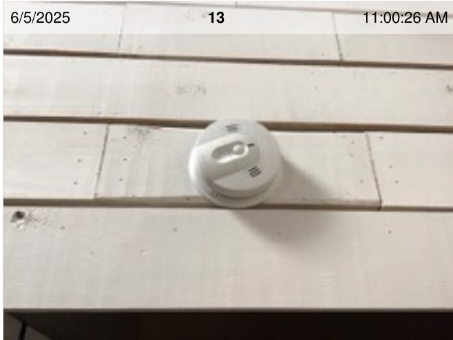
Wireless Smoke/CO Combo Smoke Alarm (mfd 6/2022) | Smoke test: Passed | Alarm in place
