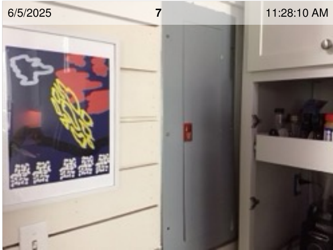
Electrical Breaker Panel
