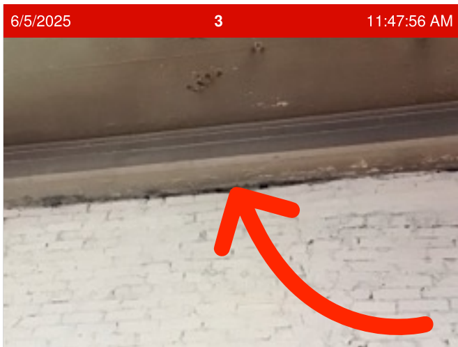
Ceiling | Major cracks in ceiling | Tenant explained that there is sunlight being able to get through the cracks just above their bedroom area
