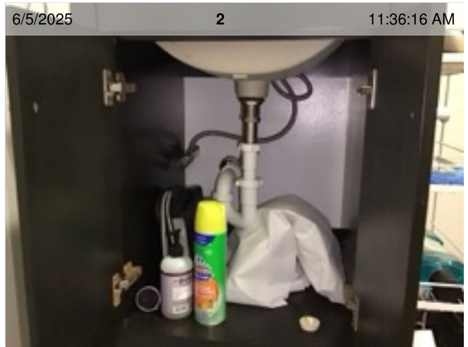
Cabinet Under Sink
