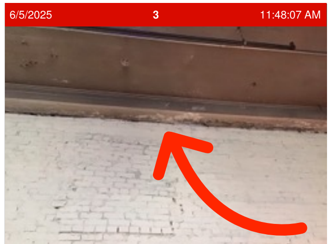
Ceiling | More of ceiling cracks in the roofline
