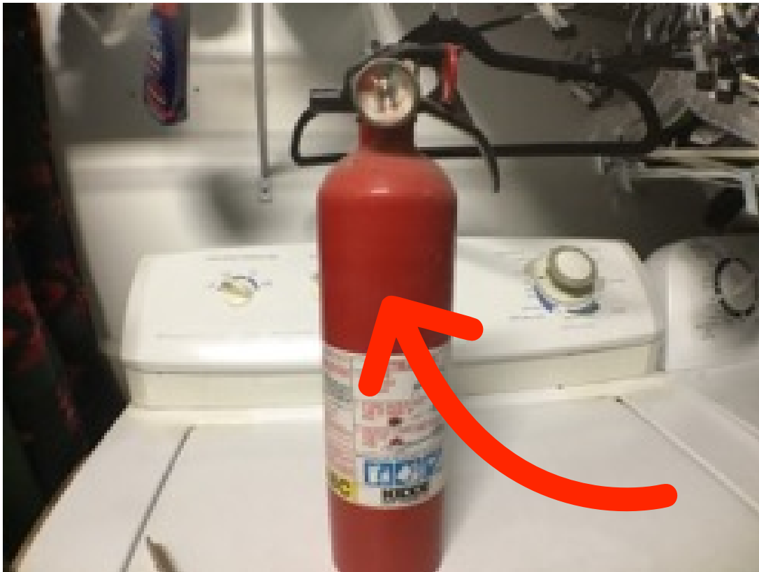
Laundry Room Fire Extinguisher Empty extinguisher
