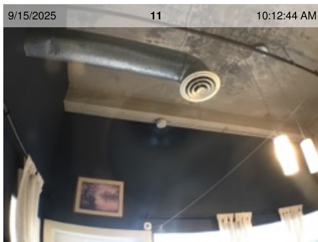
Inaccessible Smoke Alarm | Smoke test: Not tested | Alarm in place | Obstructed access to alarm
