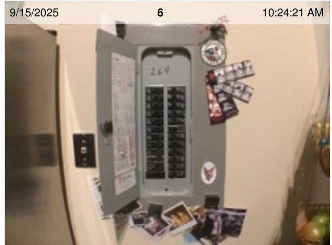
Electrical Breaker Panel
