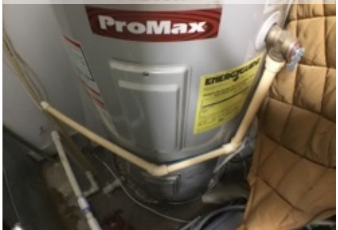
Electric Water Heater | A.O. Smith | Water heater (with expansion tank if present)
