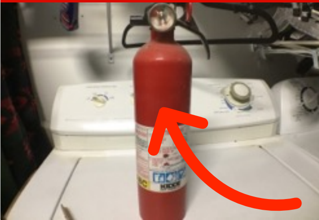
Fire Extinguisher | Empty extinguisher
