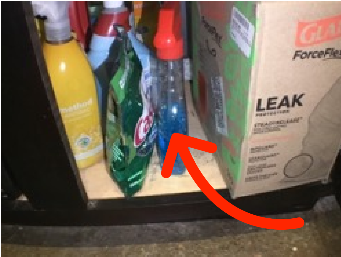
Kitchen Cabinet Under Sink The base of the cabinet is discolored.
