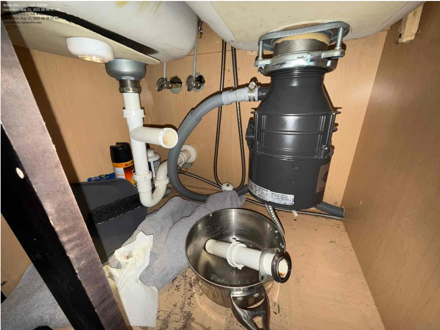
Reroute hose so no backwash to dishwasher
